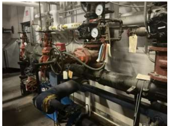
24 - FIRE SUPPRESSION SYSTEM
