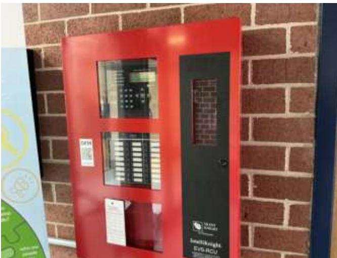
23 - FIRE ALARM PANEL
