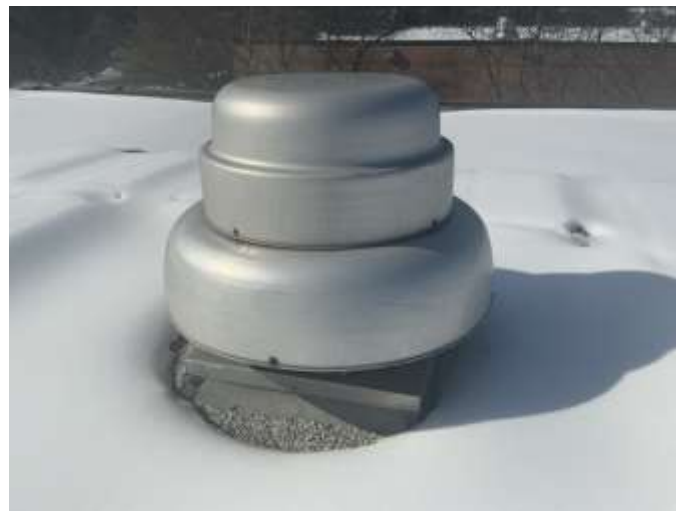
18 - TYPICAL EXHAUST FAN
